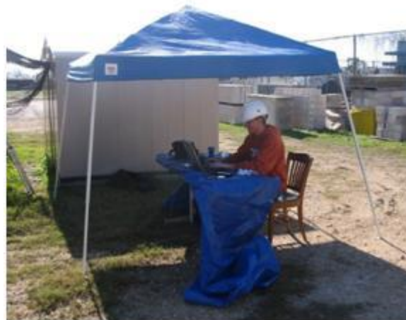
Figure 10. Remote load cell monitoring.
